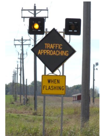
Minor Road Warning System
